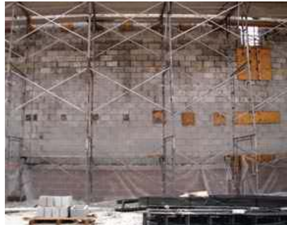
Figure 3 CMU wall section with inspection ports are time consuming and expensive.
